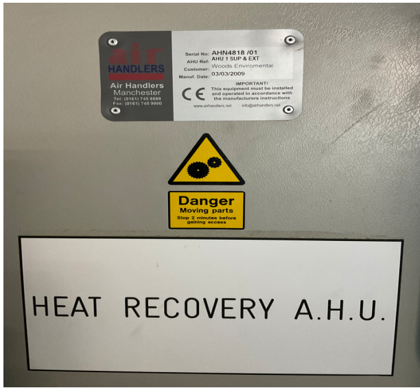
Heat recovery AHU
