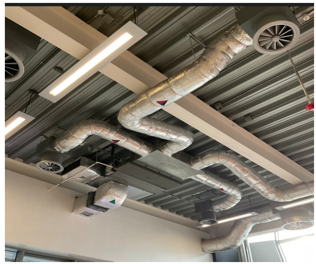
Fan coil unit with swirl diffusers
