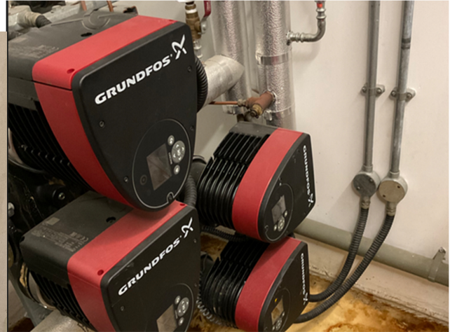
Heating system distribution pumps
