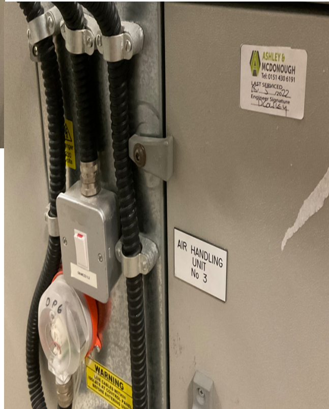
Air handling unit
