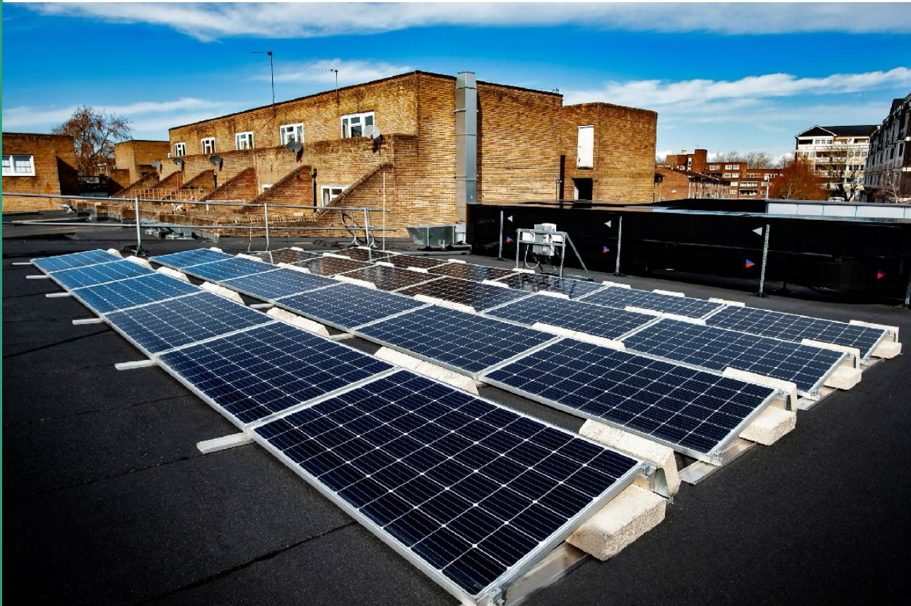
Solar panels installed on the roof of a building owned by the Royal Borough of Greenwich Council
