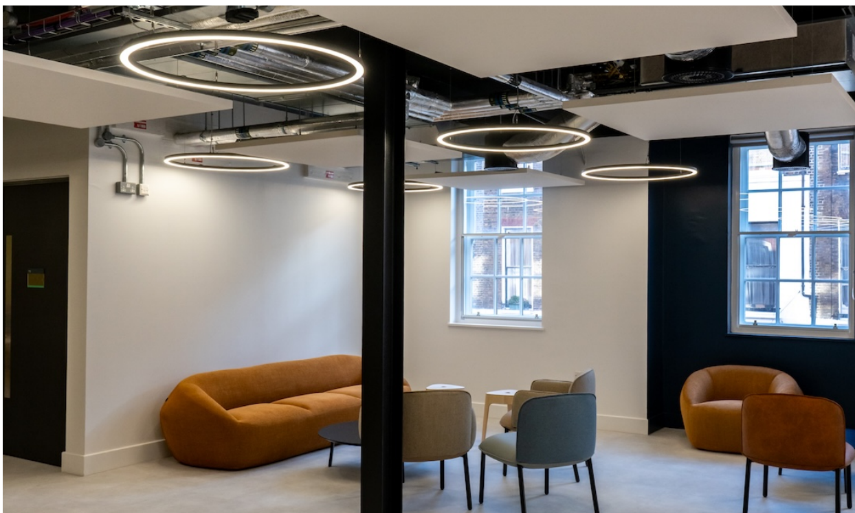
New energy-efficient lighting installed at the London School of Health and Tropical Medicine
