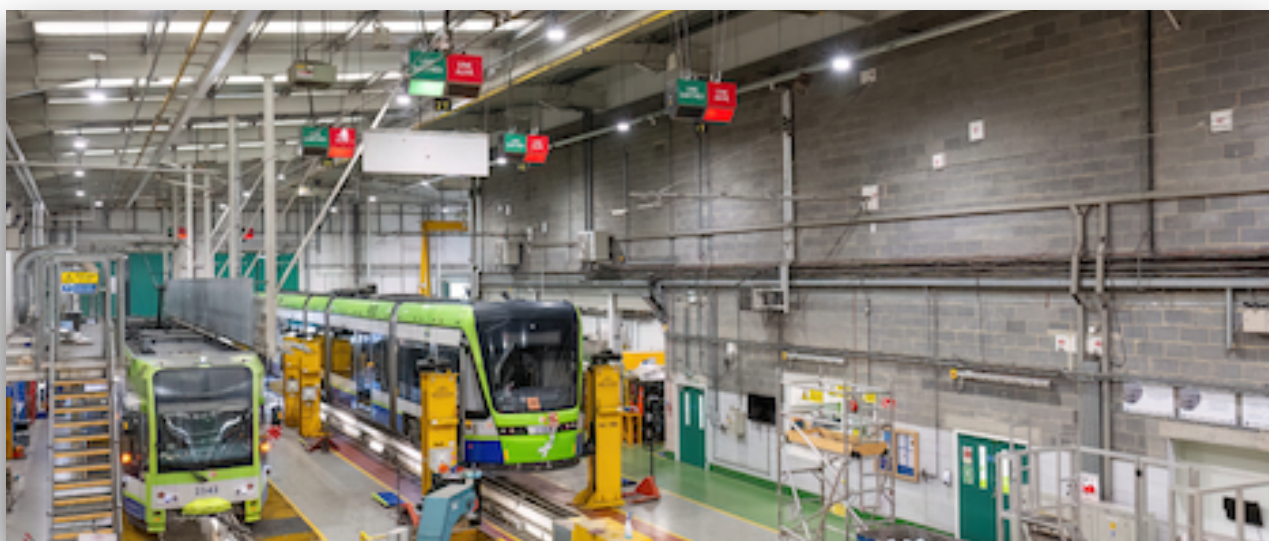
Transport for London's Therapia Lane tram depot where funds from the Public Sector Decarbonisation Scheme were used to install energy efficiency measures which are forecast to save around 183 tCO 2 e a year.
