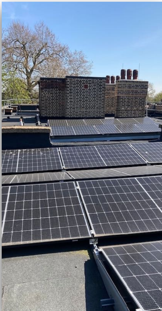
Solar panels installed on the roof of social housing in Lewisham in south London.
